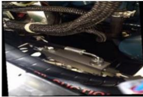
New position of over centre valve
